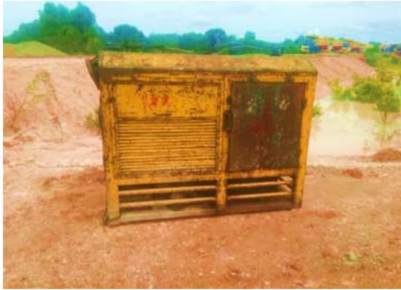
Gambar 3.5 Generator Set (Genset)
